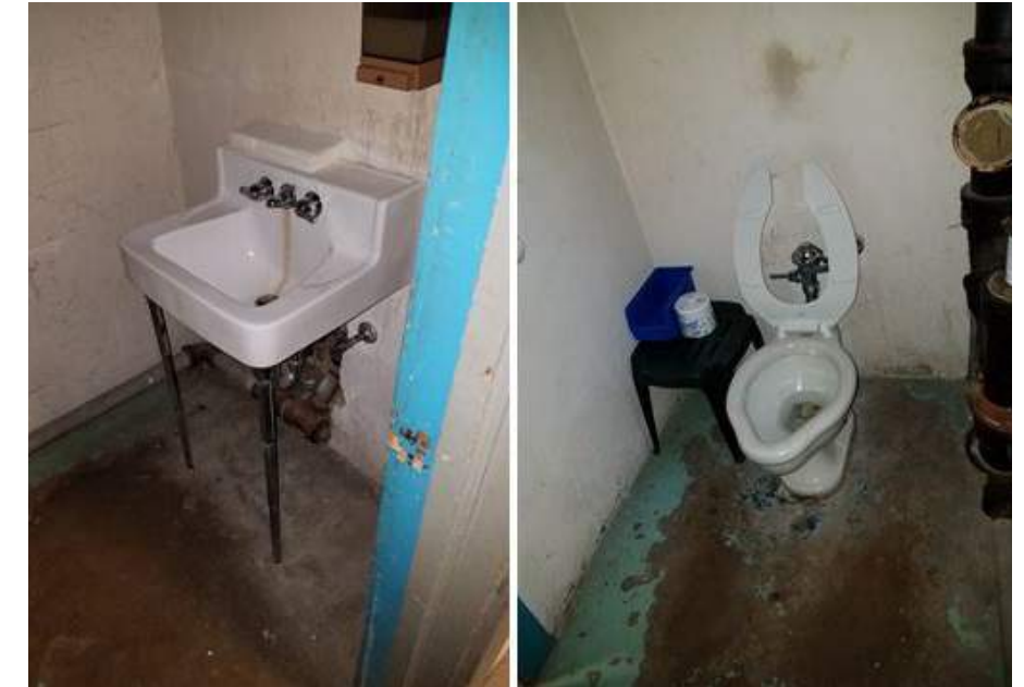
Lavatory and toilet original to building having reached their useful life
