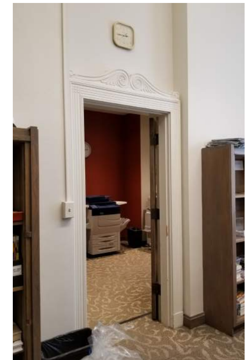
Current condition of the original north wall. Opening height was increased, destroying the rest of the large central north wall mural.
