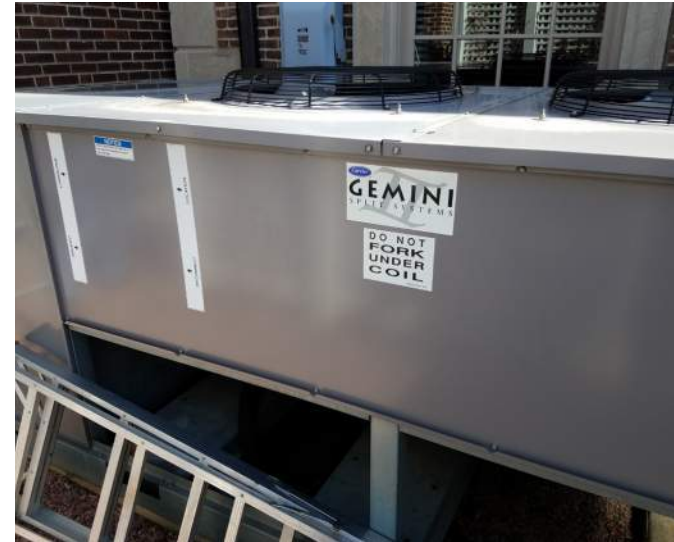
Large capacity air cooled condensing unit (unit shown in previous picture with cooling tower)
