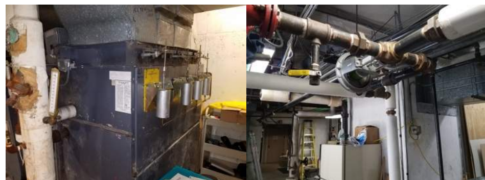
Typical pneumatic damper actuators on AHU Three way pneumatic control valve
