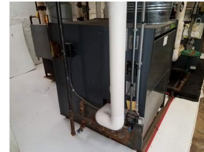
Slightly Newer Hot Water Boiler
