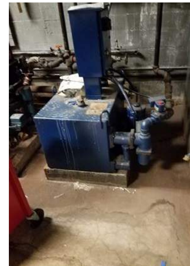
Steam Condensate Transfer Unit
