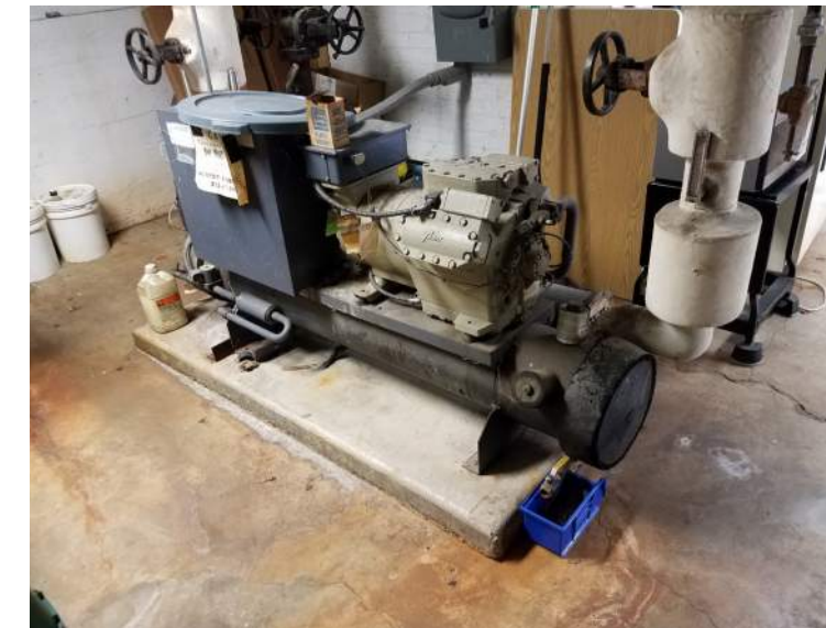
Trane water cooled chiller
