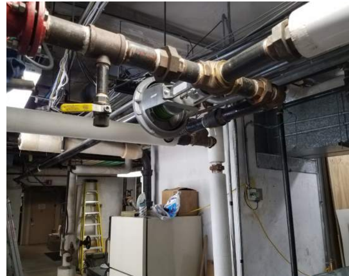
Piping missing insulation
