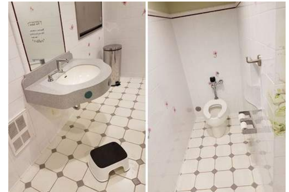
Newer plumbing fixtures in good condition
