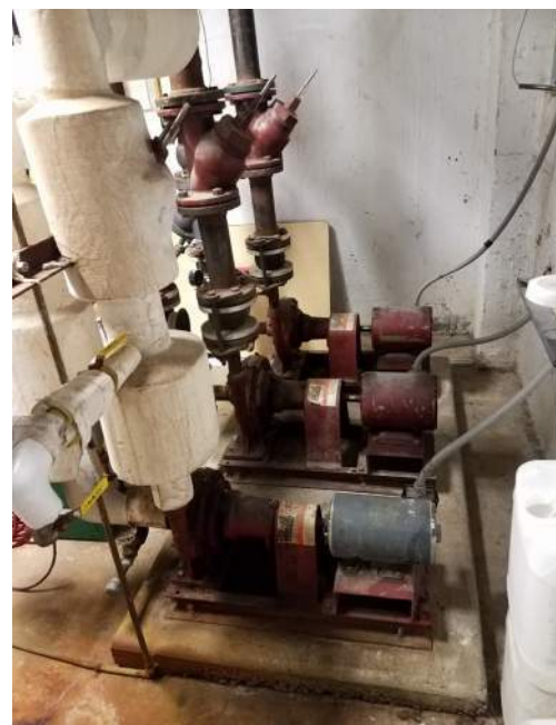
Second set of hot water pumps and chilled water pump
