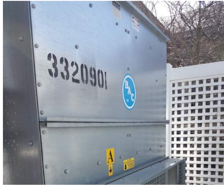
Cooling tower and air cooled condensing unit
