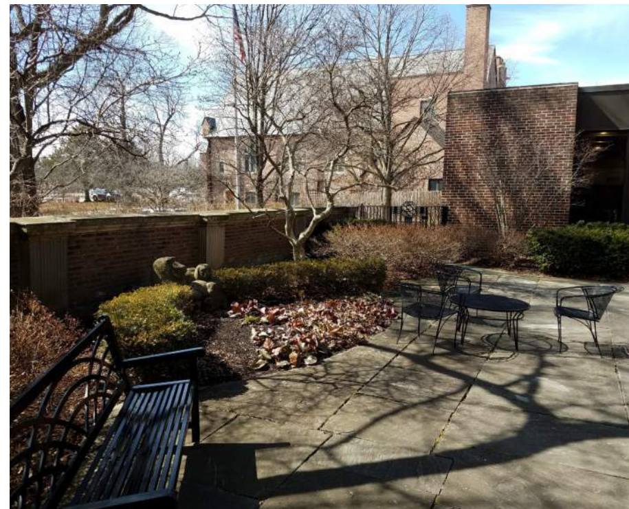
Garden walls that show signs of settlement
