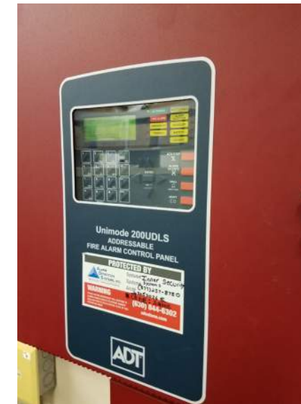
Existing Fire Alarm Control Panel
