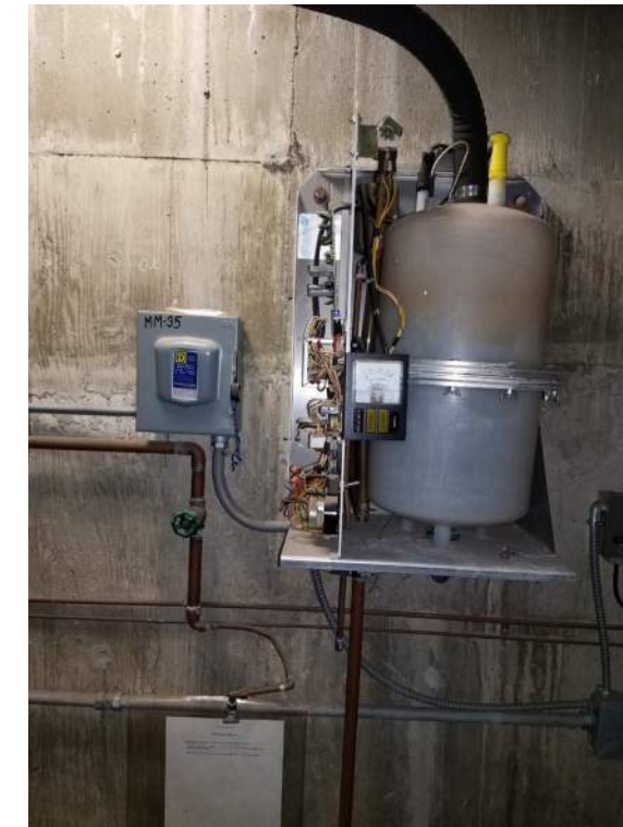
Canister type humidifier abandoned in place
