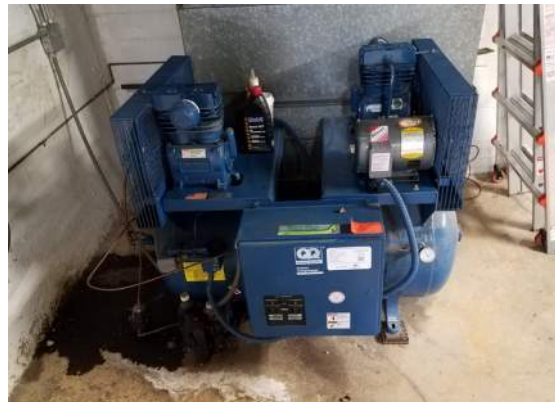
Pneumatic control air compressor in good condition
