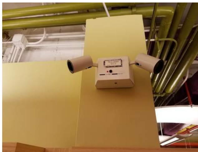
Emergency Battery Lights
