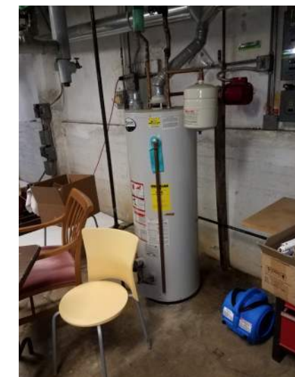
50 gallon, 40,000 btuh gas water heater
