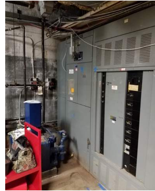
Main Electric Service Switchboard
