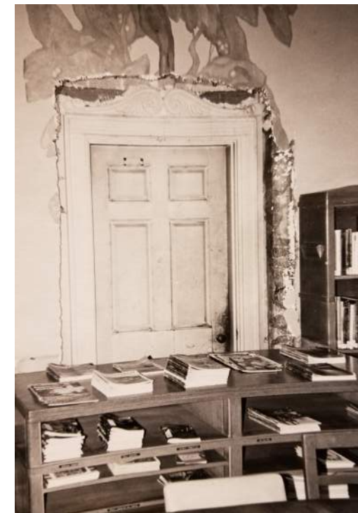
North wall - door was added later, probably when the Garden Room was converted to a music room. Insertion of the door destroyed portions of the mural.
