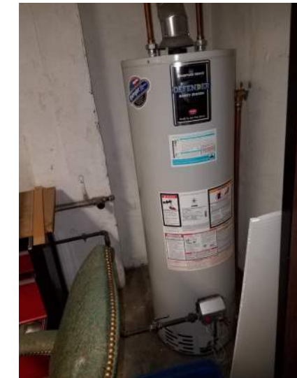
40 gallon, 40,000 btuh gas water heater
