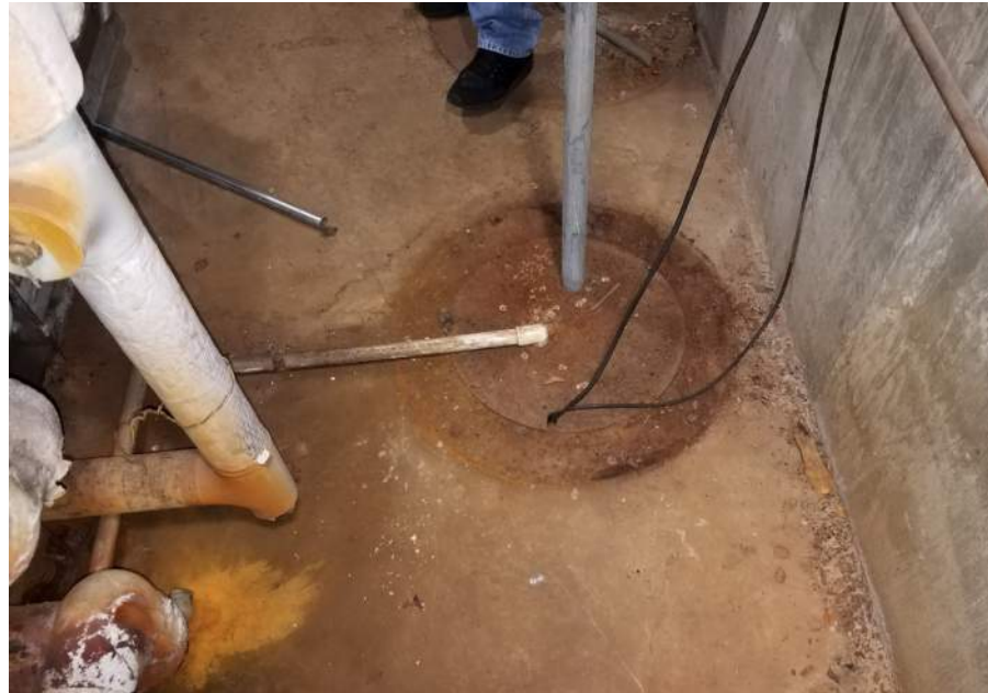
Typical foundation ground water sump pump
