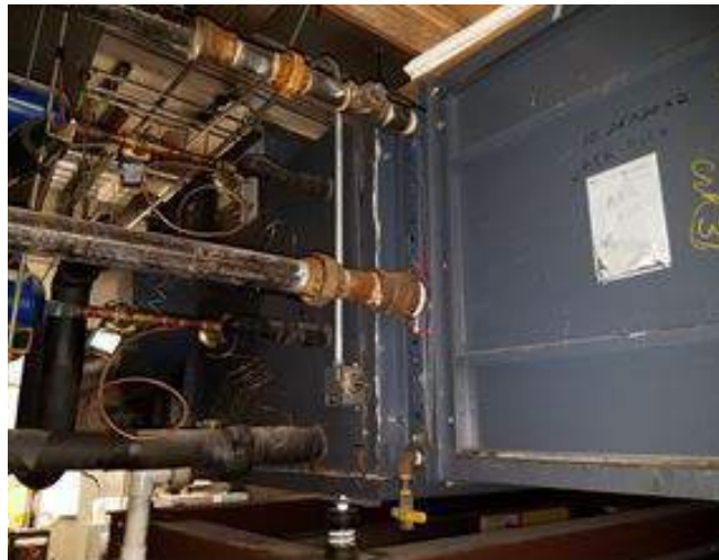
Typical AHU's with DX cooling coils. One old and one fairly new
