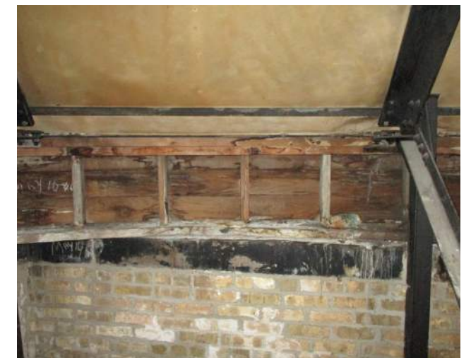
Poor condition of wood cricket wall below dome structure
