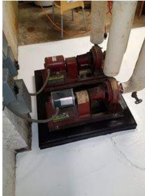
One set of hot water pumps
