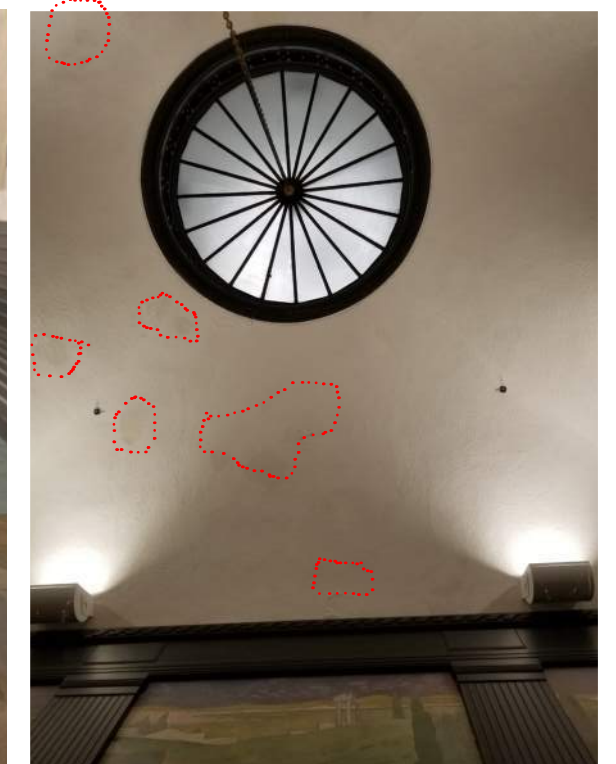
Plaster ceiling staining (viewed facing west wall) occurs on the south side of the room and which corresponds with observed mural damage.
