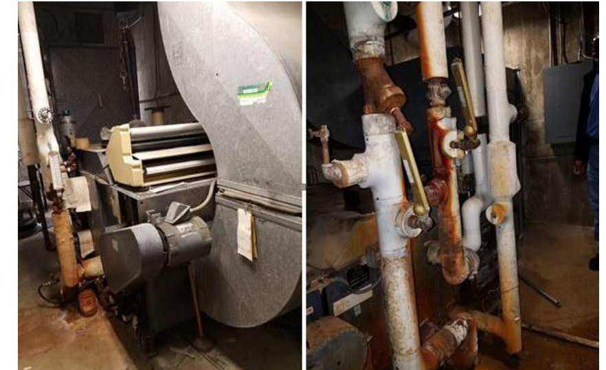
Single zone air handling units with hot and chilled water piping connections
