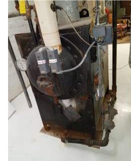
Original Hot Water Boiler
