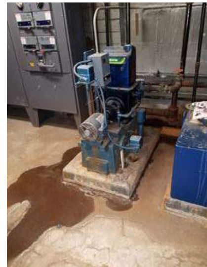
Steam Boiler Feed Unit
