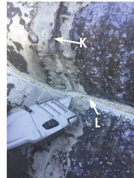
Sealant at joint in ornamental copper
