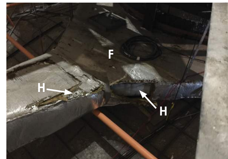
Deteriorated duct insulation
