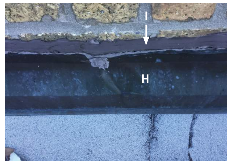
Damaged flashing and sealant patch at north roof
