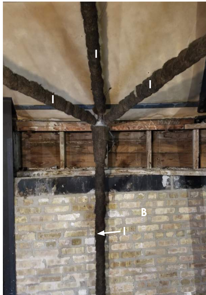
Skylight condensate piping collects on the north side of the attic
