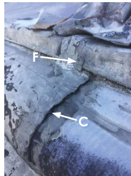
Solder joint at roof base
